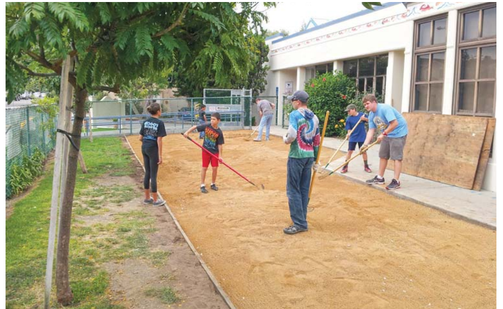
Before any construction could be done, the Scouts were responsible for removing 6-cubic feet of soil, removing grass and weeds, coordinating with city closure of Richmond St. and laying landscaping fabric on the ground.
